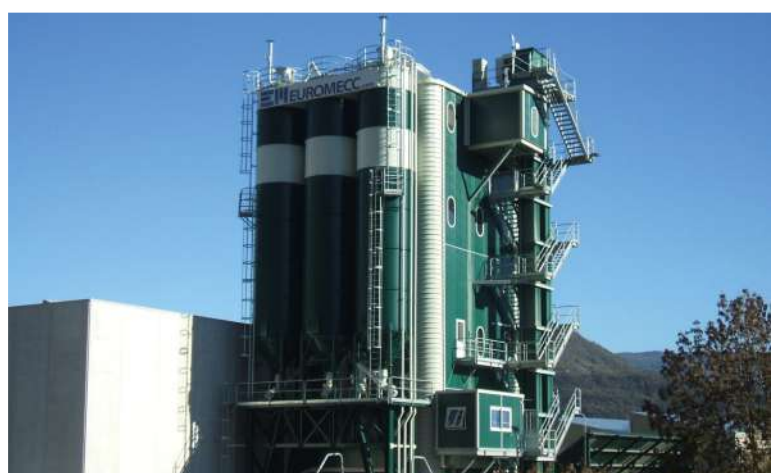
Trento, Italy: Tower plant for pre-cast and readymix
