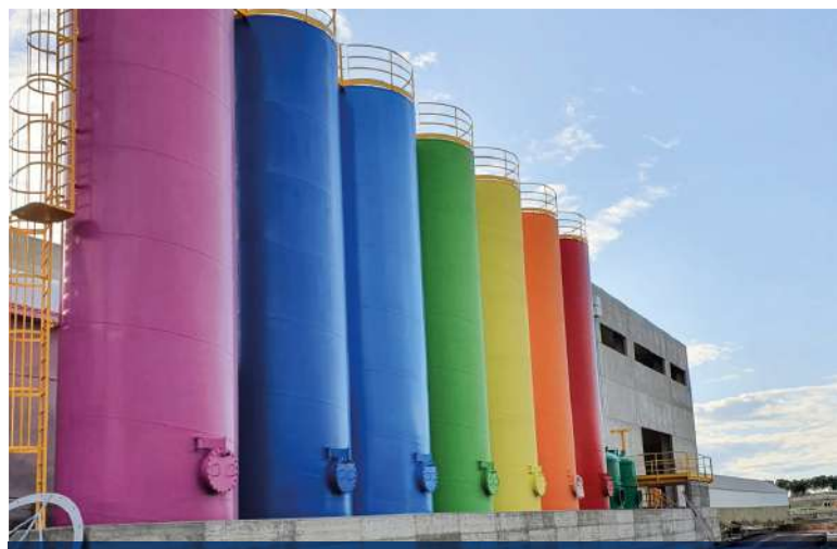
Catania, Italy: Storage tanks for waste treatment
