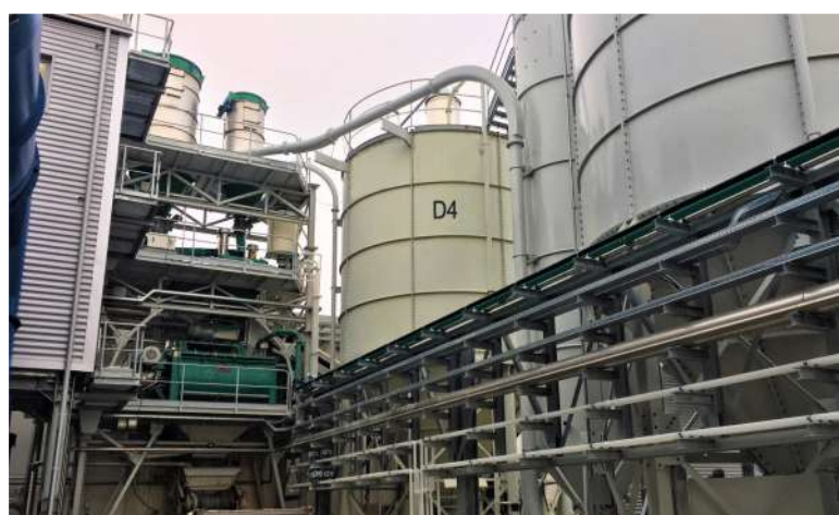
Foggia, Italy: Waste treatment plant
